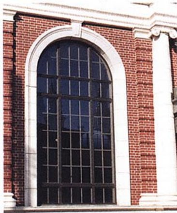
Custom-designed storm windows are available for very large openings, as seen here at Covington Station in Covington, KY.
